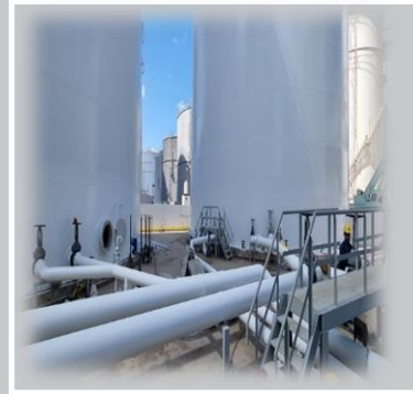
Above Ground Pipeline
